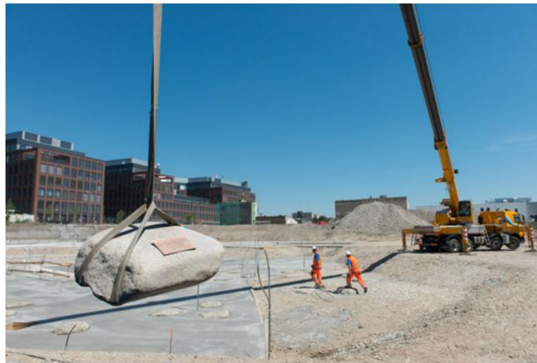
Laying of the 600kg foundation stone of the Sky Park project by Zaha Hadid. (Source: Jana Liptáková)
